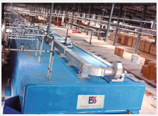
Moisture Control System
