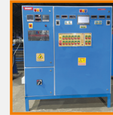
Auto Speed PLC Control Panel & Separate Desk Gear Drive System
