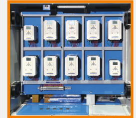
VFD for Blower to Save Power
